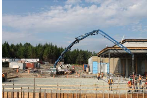
Figure 1: FRP-reinforced concrete tank, Qc, Canada.
